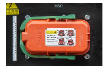
The MSD maintenance switch
