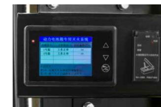
Automatic battery fire extinguishing devices
